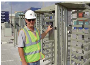
RTD-15.1 turnstile at Jebel Ali port in Dubai city, U.A.E.
