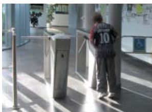
TTD-03.1 turnstiles at Laugardalslaug Geothermal Swimming Pool in Reykjavik, Iceland
