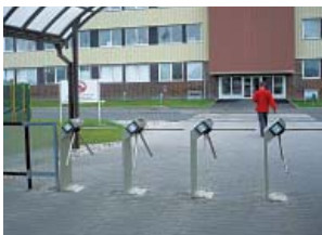
TTR-04W turnstiles at Bosch and Siemens factory in Michalovce, Slovakia
